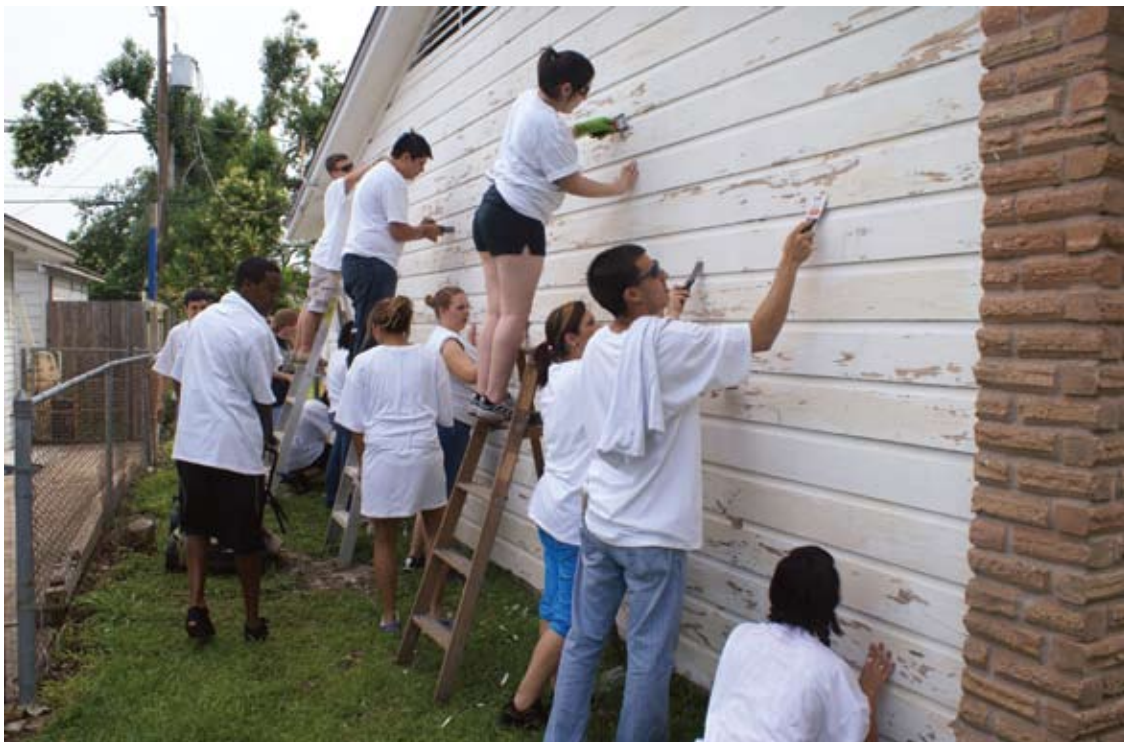
Pasadena Memorial High School students prep an exterior wall prior to giving it a new coat of paint.
