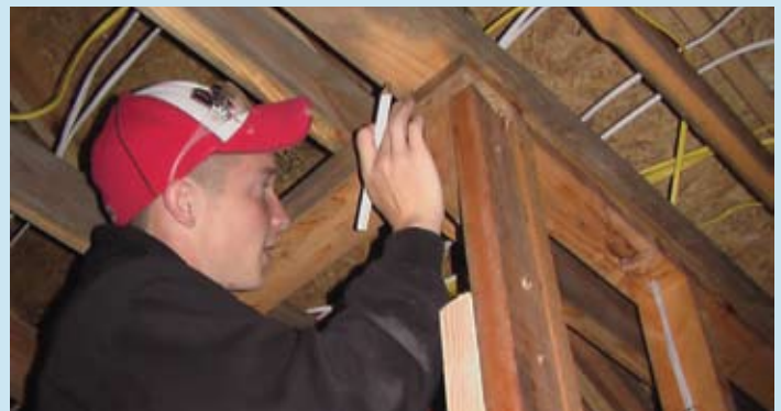
Kriz Ledbetter of Birdville High School works on an interior wall of a house.
